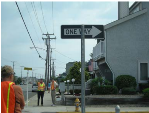
PICTURE 7: ONE (1) ONE-WAY SIGN MOUNTED INSTEAD OF BACK- TO-BACK MOUNT, NON- BREAKAWAY POST AT PRIMROSE AVENUE
